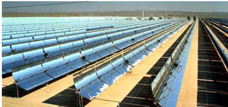
Solar Electric Generating System, Kramer Junction, CA
